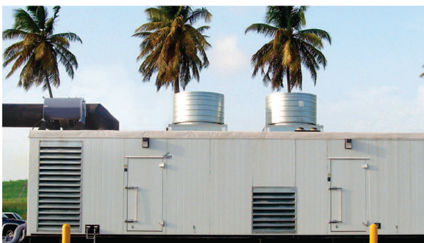
GE's genset provides power on the island of St. Kitts
