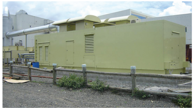
GE Transportation's gensets power a factory in Fiji
