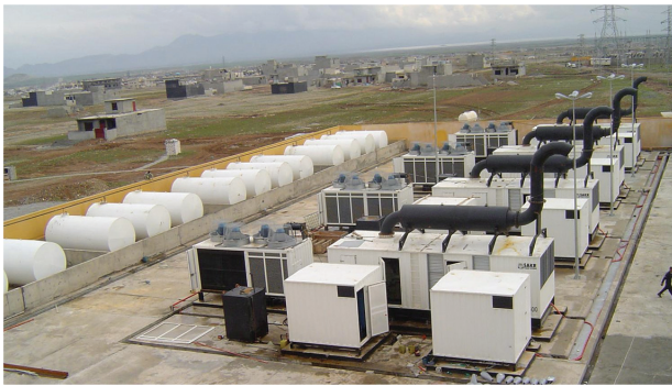
Enclosed gensets power the grid in Northern Iraq
