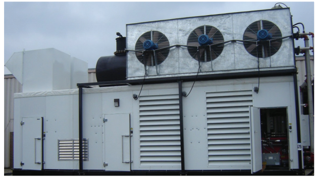
An enclosed genset provides power in New Orleans
