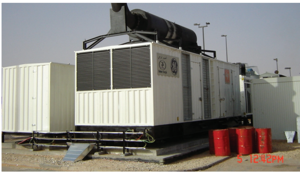
Enclosed gensets installed in Algeria
